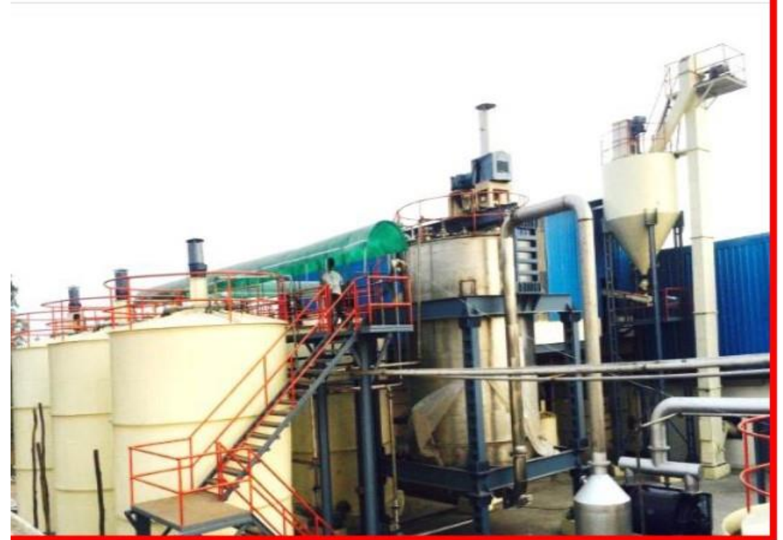
View of OPM - Onsite PCC Plant
